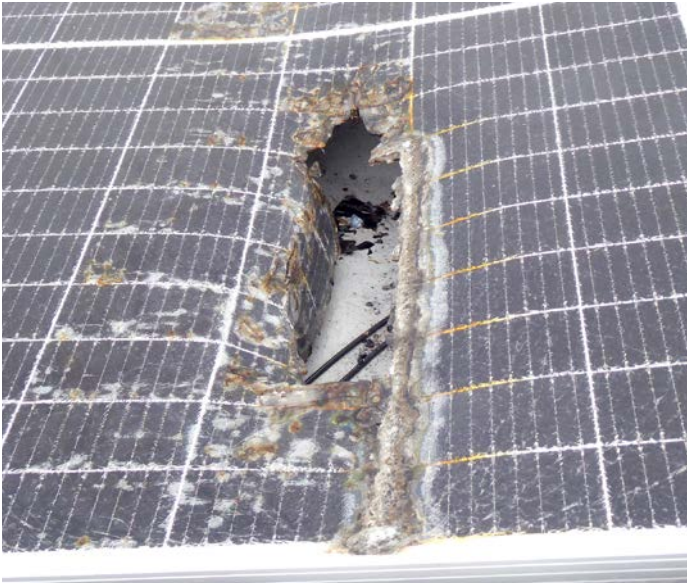
The back sheet material in this module was obviously a bad choice.
